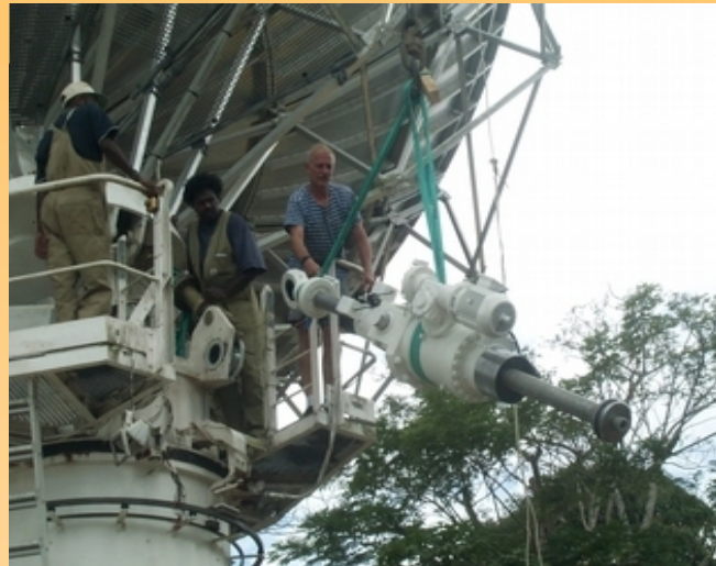
ALCATEL Antenna in Vanuatu
